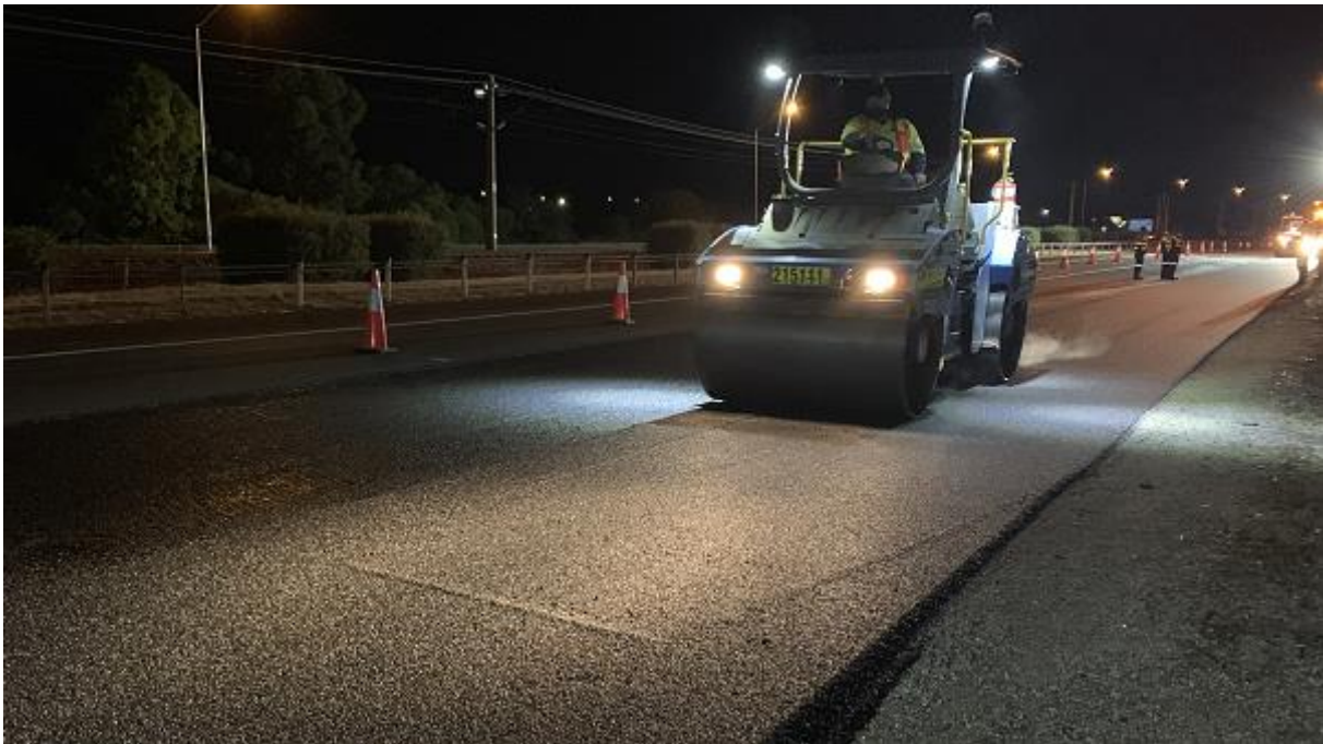
Figure 5.9: Compaction with vibrating steel wheel roller of eight tonne mass on shoulder, Kwinana Freeway
