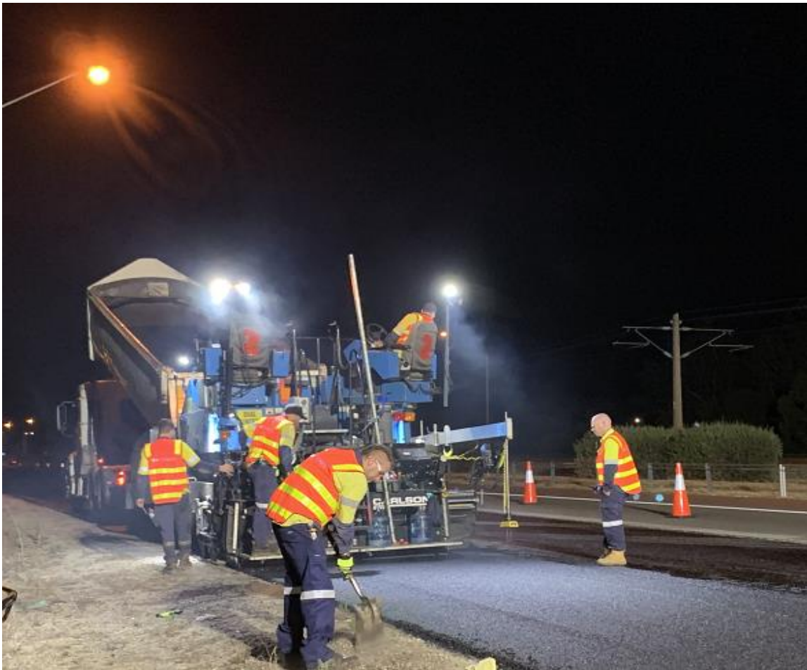
Figure 6.1: Visible fuming with load of mix tipped into paver (1 st truck on site)
