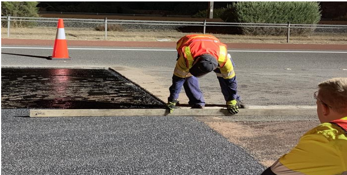
Figure 5.8: Attention given to level of terminal transfers joint on shoulder, SLK 25.46, Kwinana Freeway
