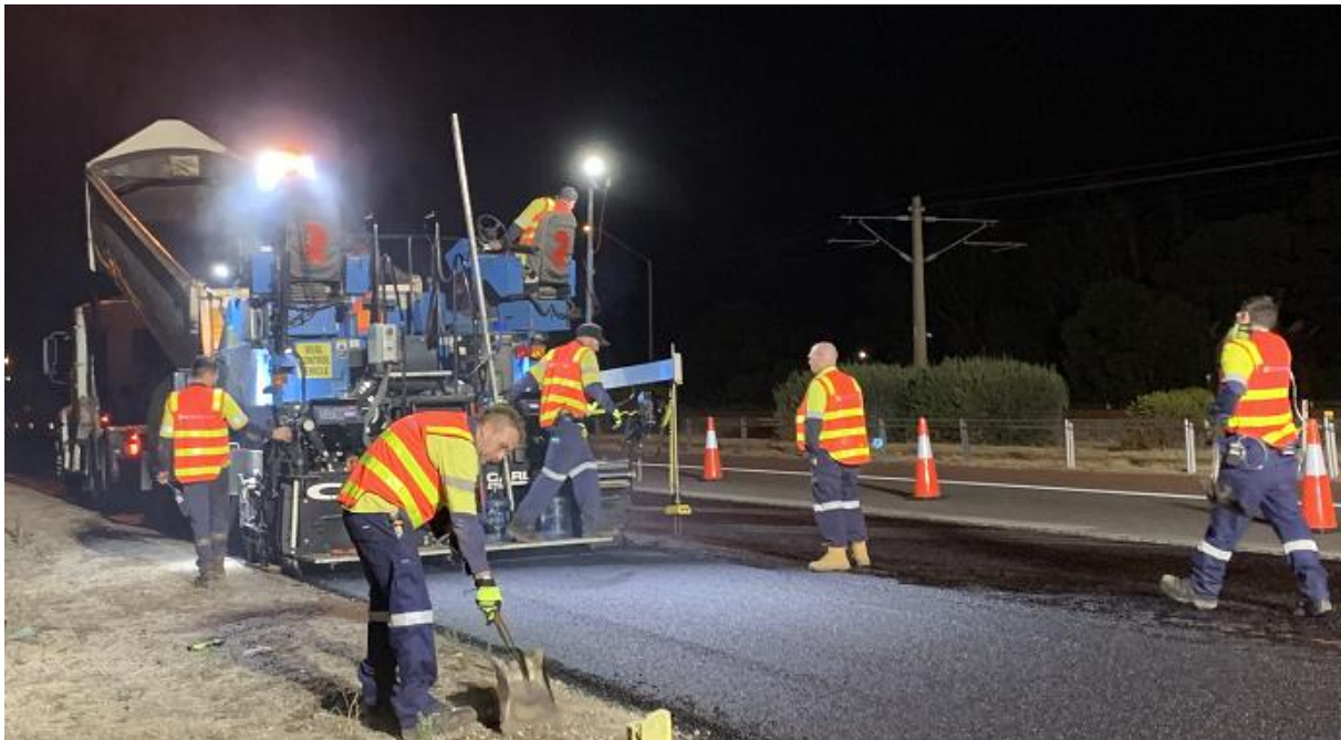
Figure 5.7: Placement of CRM OGA (alternative PSD) commencing on shoulder, SLK 25.46, Kwinana Freeway
