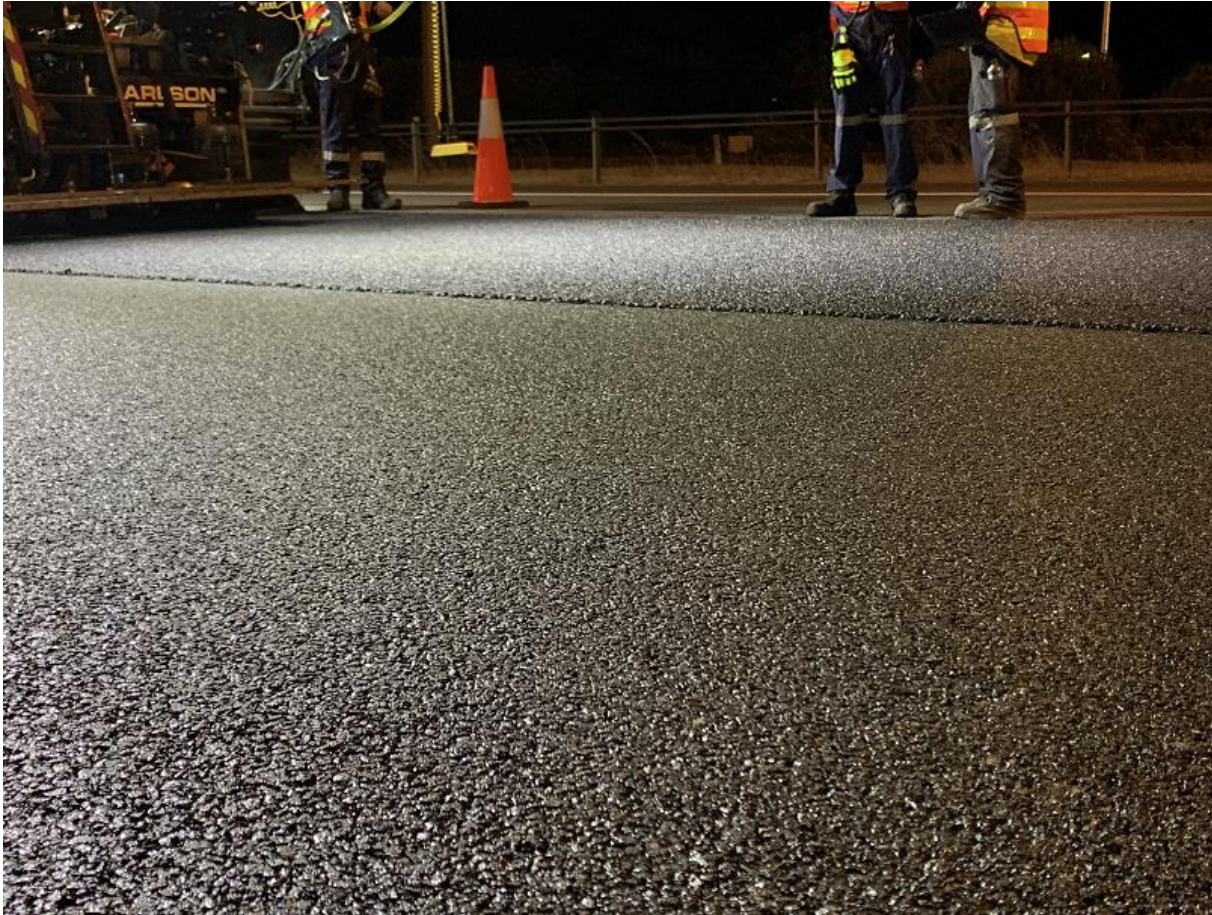
Figure 5.11: Compacted CRM OGA (alternative PSD) on shoulder and uncompacted pull on L2
