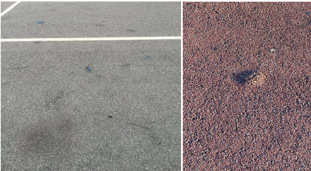
Figure 2.4: Blistering of surface above a CRC pavement (left – car park, right – shared path)
