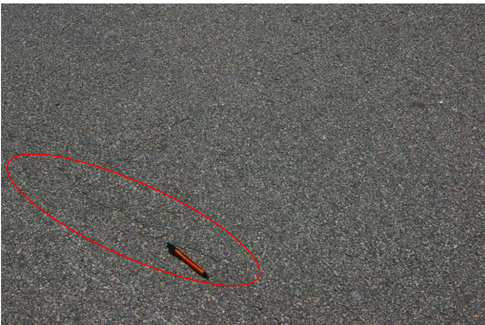
Figure 4.3: Hairline cracking in the CRC section on Gilmore Avenue
