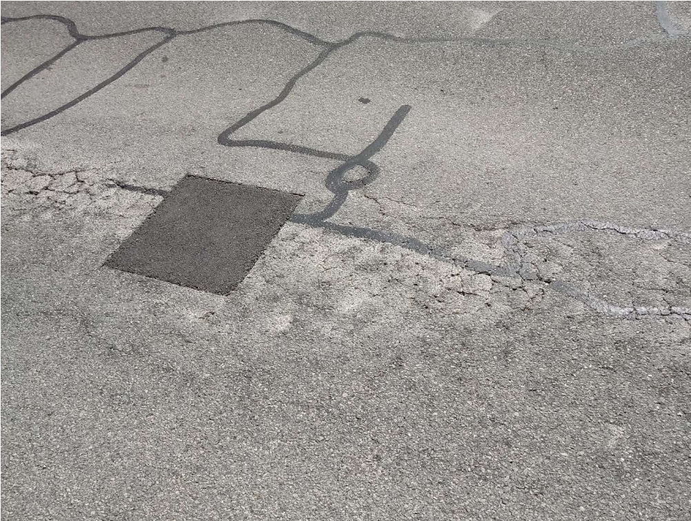
Figure 4.4: Failed section of CRC on Gilmore Avenue in 2018
