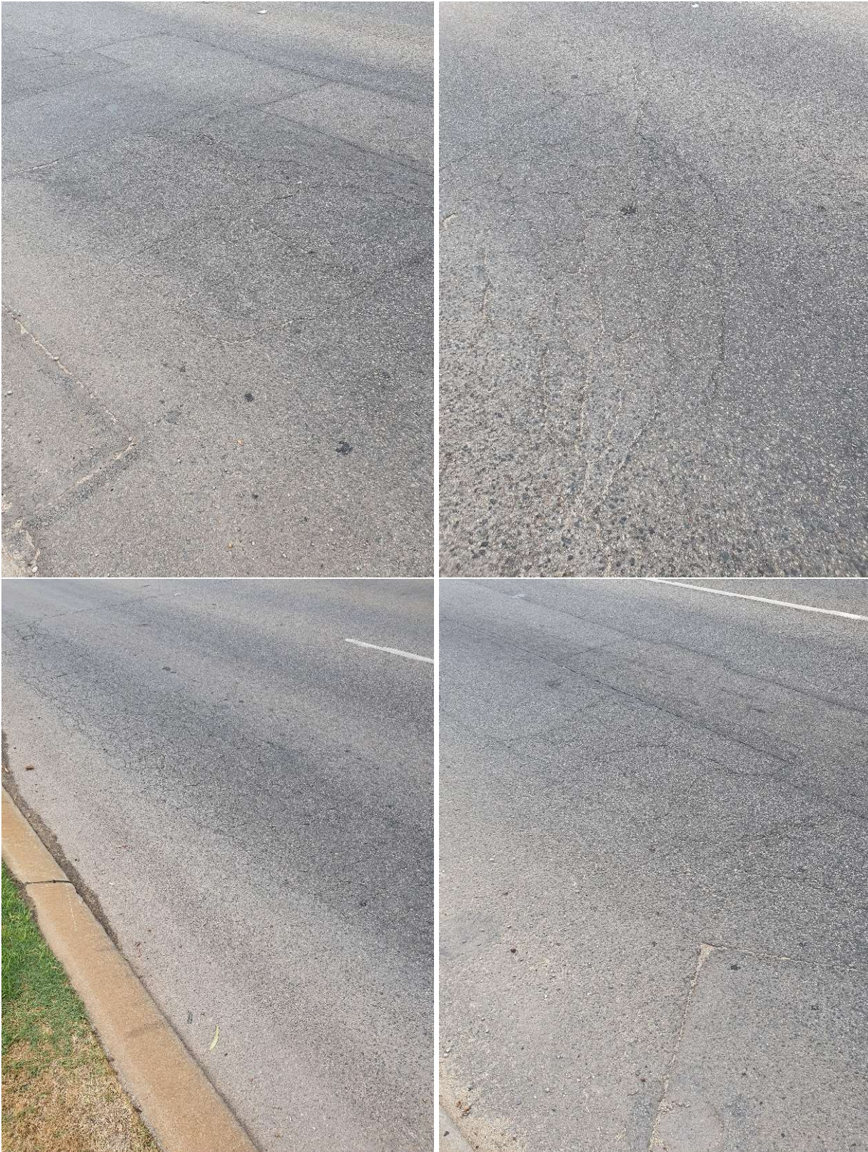
Figure 4.5: Photos of straight CRC Trial Sections 3 and 4 of Welshpool Road (taken in 2023)
