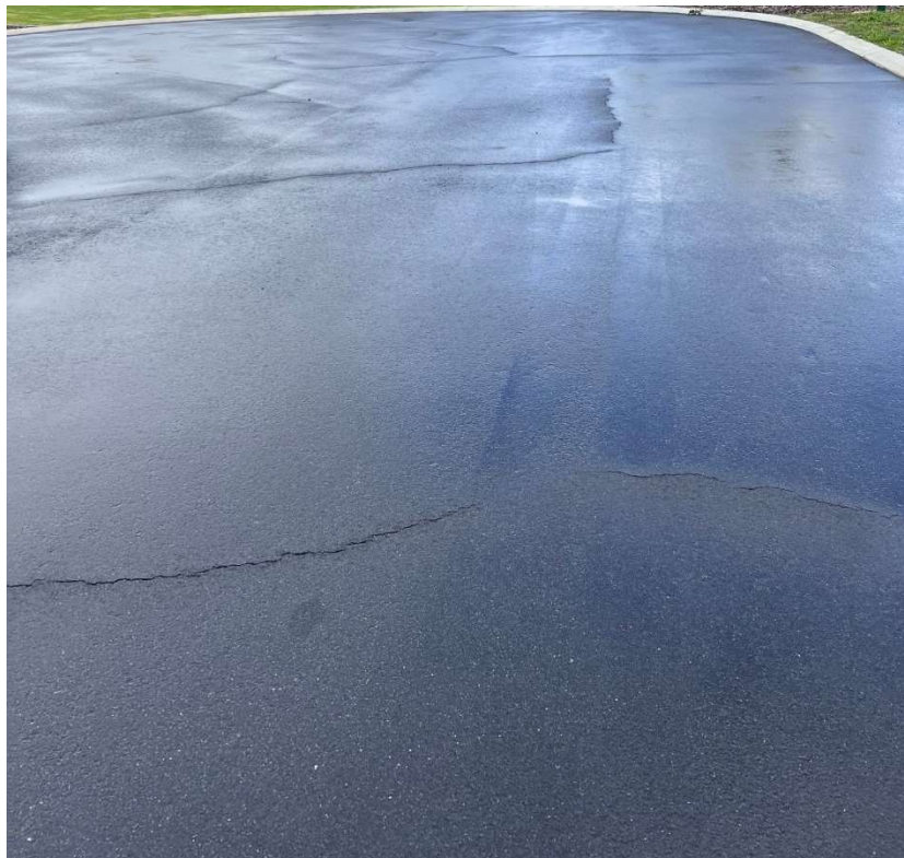
Figure 7.1: Typical block cracking on a low traffic residential street
