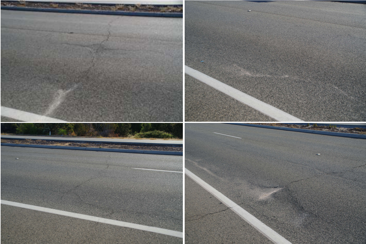
Figure 4.8: Nicholson Road pavement condition (photos taken February 2022)
