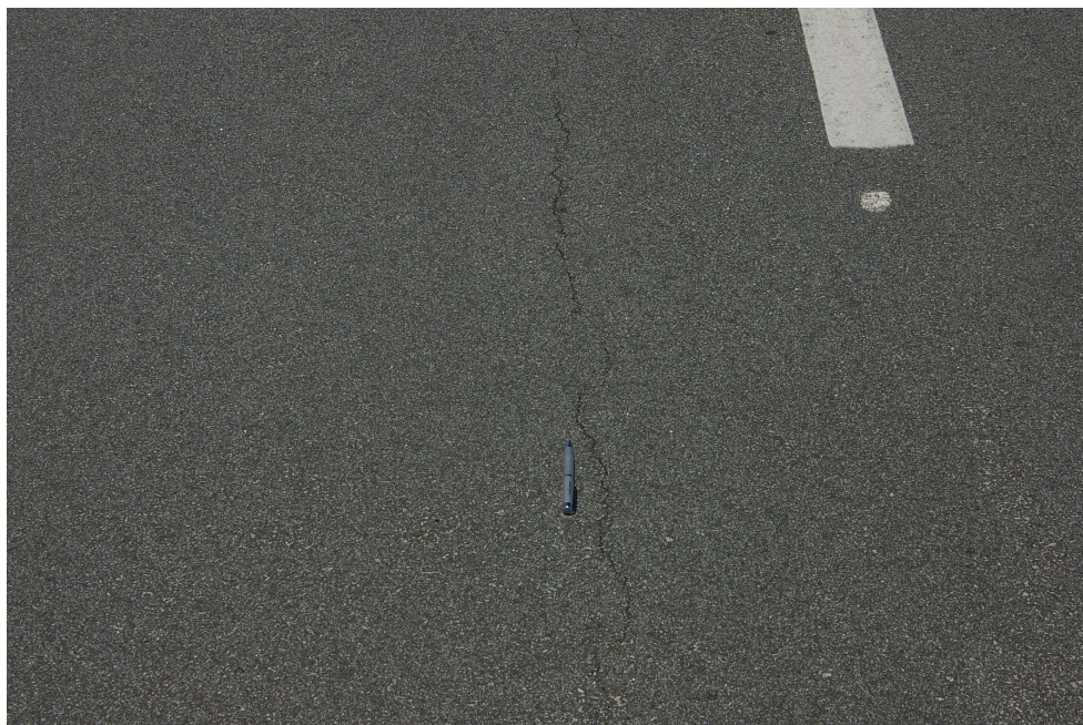
Figure 4.11: A typically more severe crack on Warton Road
