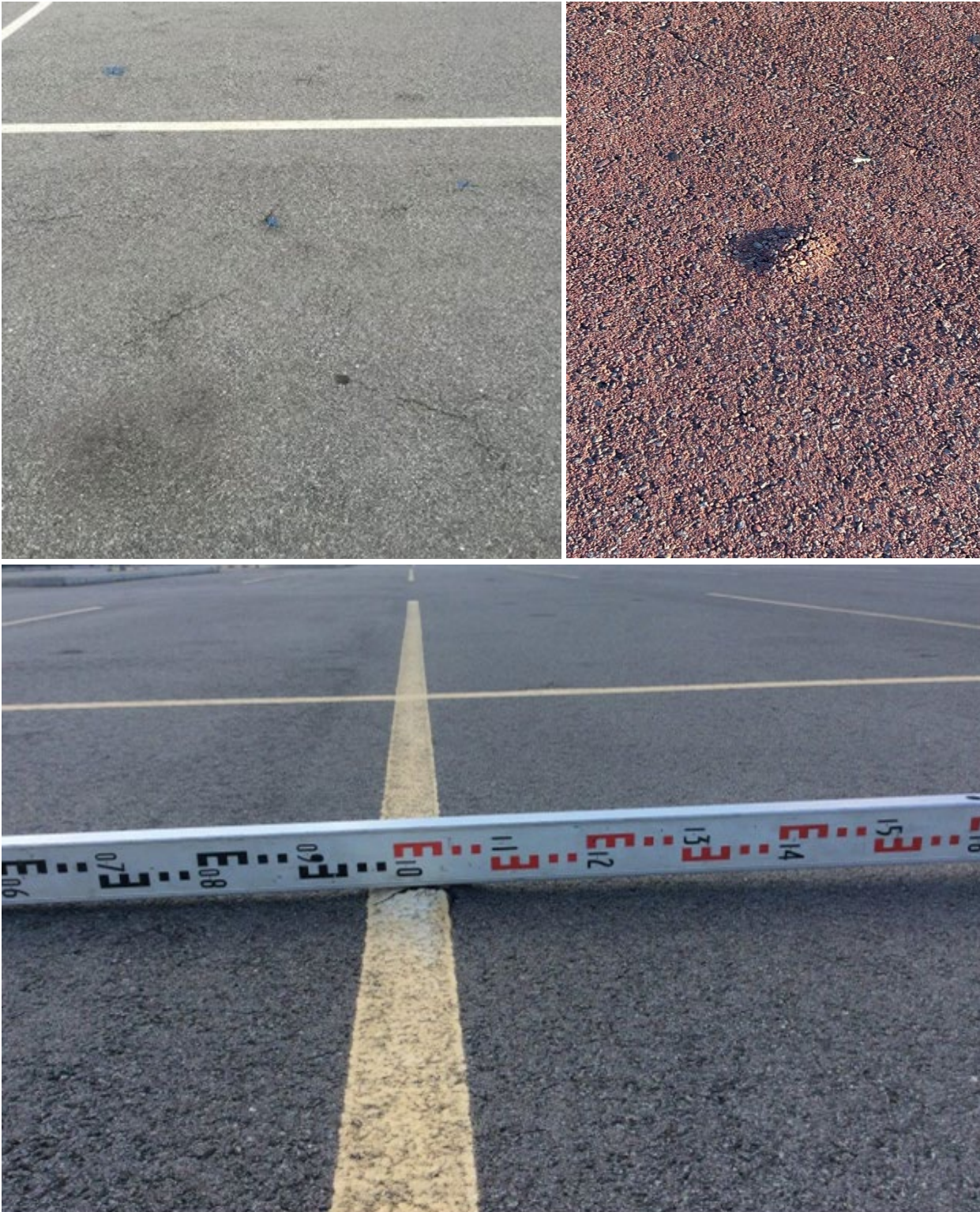
Figure 10: Example of surface blistering (left and bottom – car park, right – shared path)
