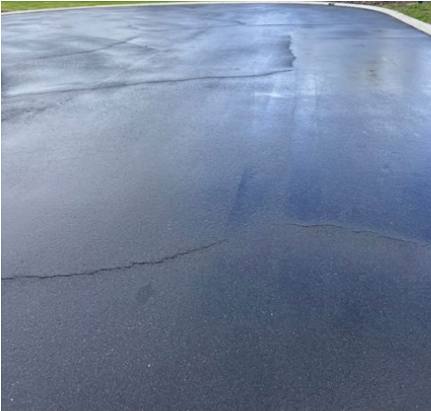
Figure 8: Typical block cracking on a low traffic residential street
