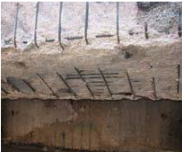
Figure 2.8: Fire damage to reinforced concrete in excess of 300 °C
