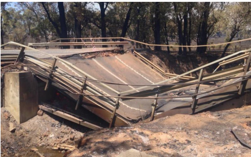
Figure 2.6: Samson Brook bridge collapse due to bushfire
