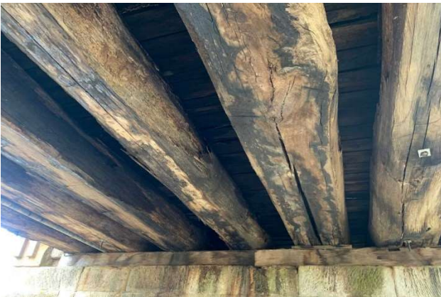
Figure 4.9: Bushfire damage to timber bridge
