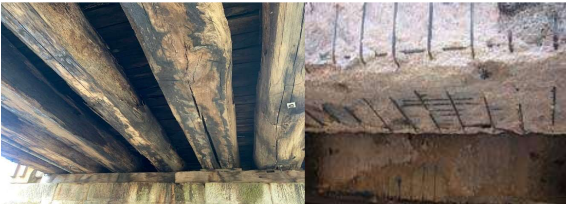
Figure 4.17: Fire damage to structures
