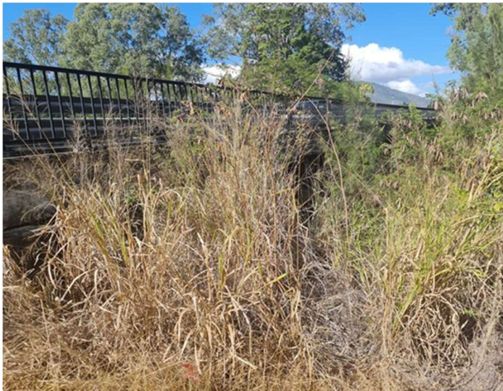
Figure 4.14: Excessive vegetation encroaching structure
