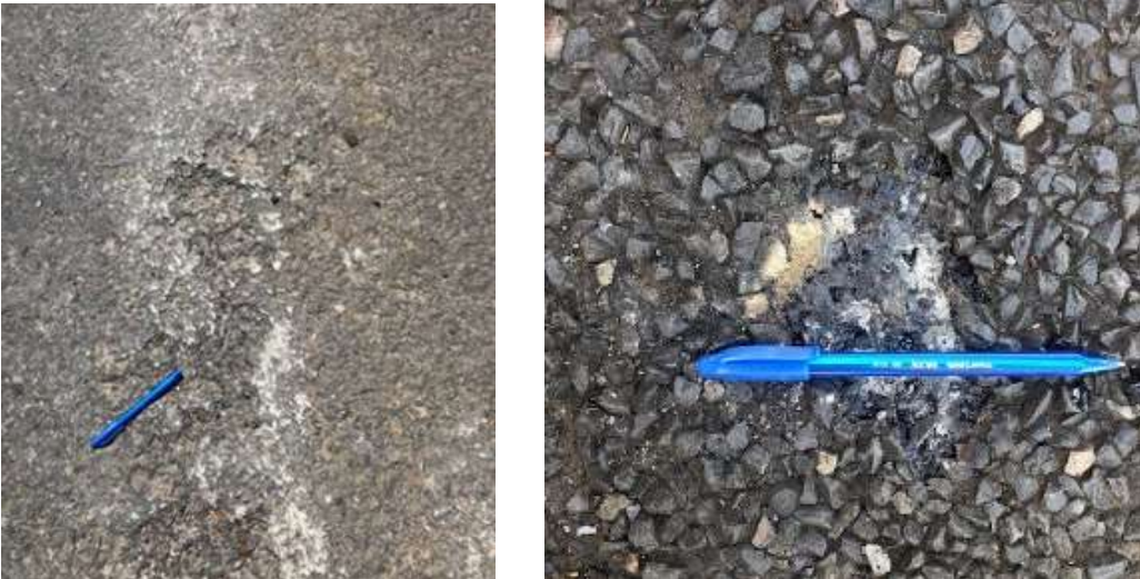
Figure 4.7: Damage to pavement materials from bushfires (left image: asphalt; right image: sprayed seal,)
