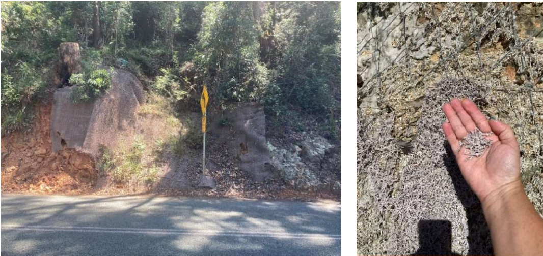
Figure 4.8: Turf reinforced matting crumbling as a result of exposure to the elements
