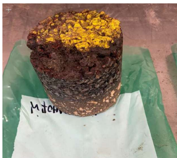
SLK 26.40 (Shoulder) – Interconnected cracks
