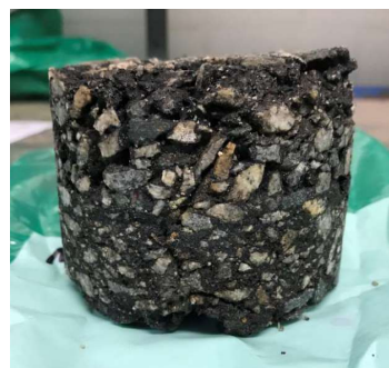
SLK 21.30 (Slow Lane) – Meandering crack
