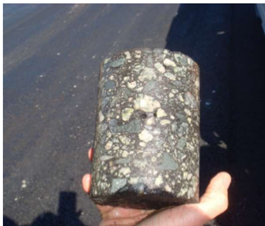
Photo 2: View of the wet core showing some of the voids at the layer interface.
