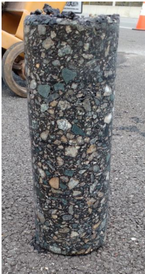
Figure A 1: Extracted core showing layers in asphalt
