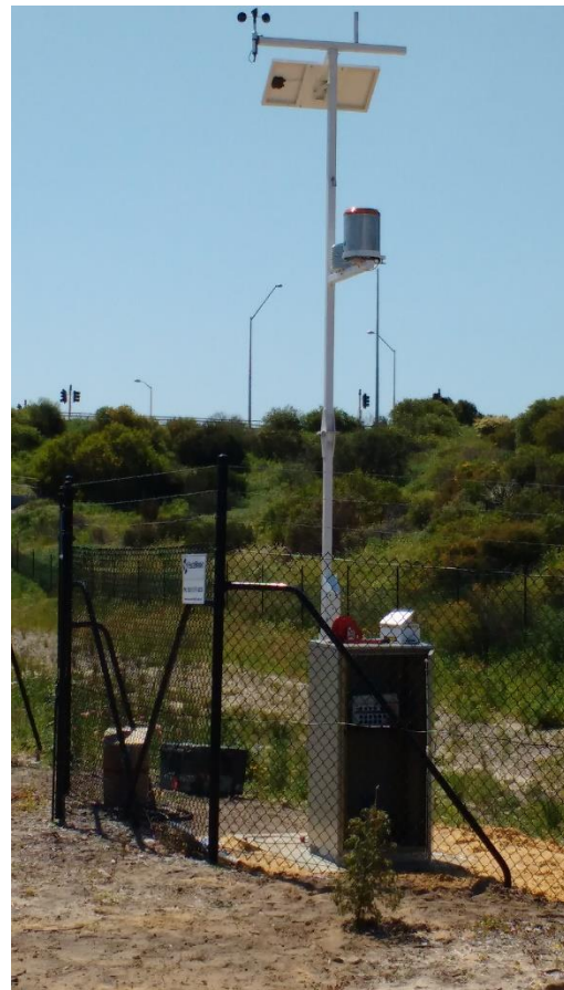
Figure A 1: Weather station after install
