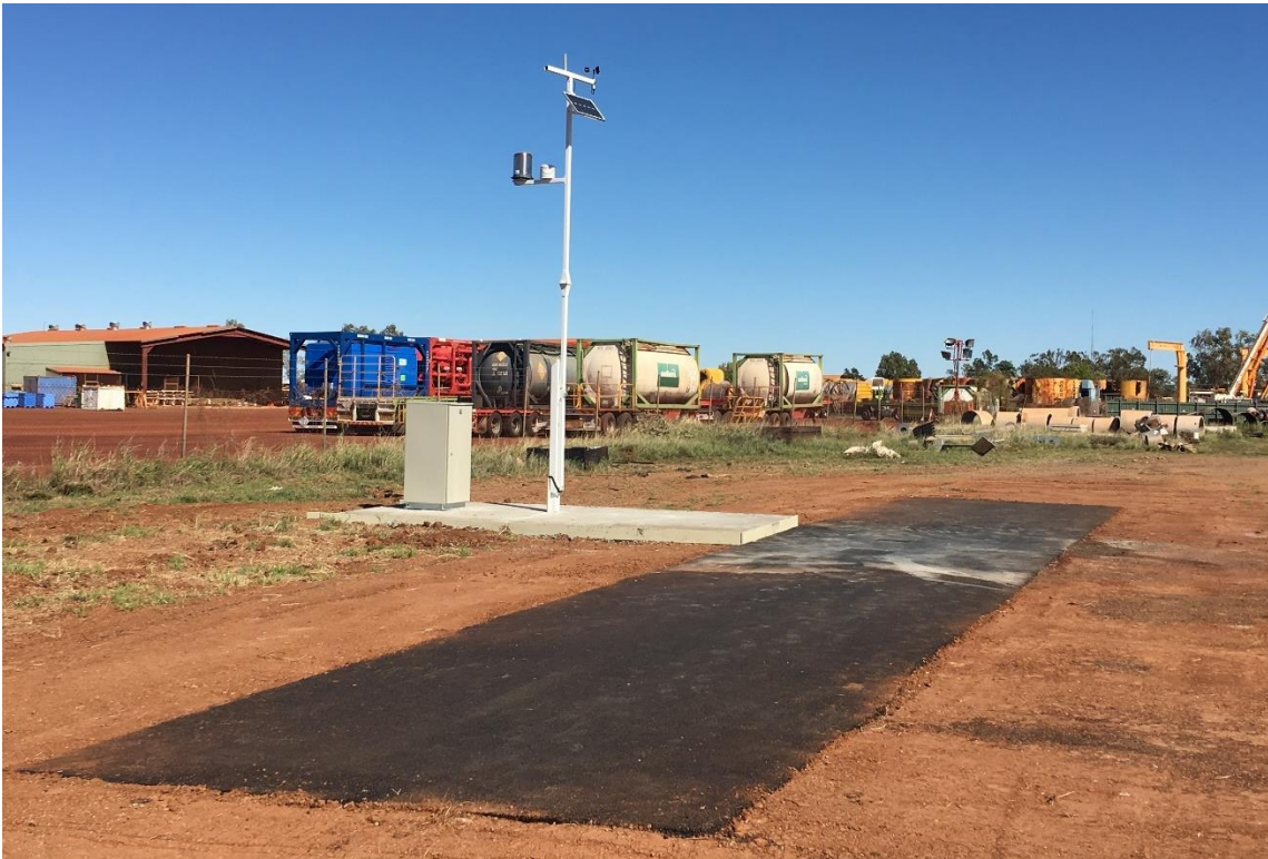
Figure 4.4: Completed installation in Karratha – June 2018
