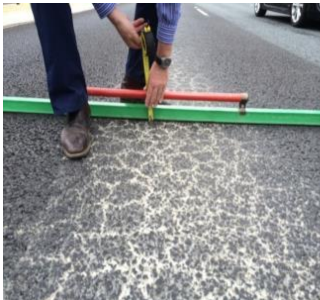
Figure 6.2: Severe pavement distress
