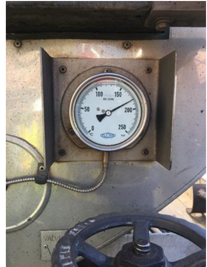
Figure 6.6: Monitoring of tank temperature
