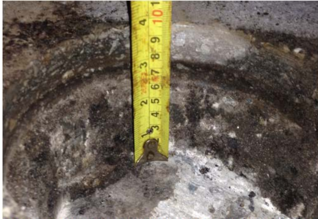
Core face of Core 3, Showing Weak and Stripped Asphalt in the Lower Layer
