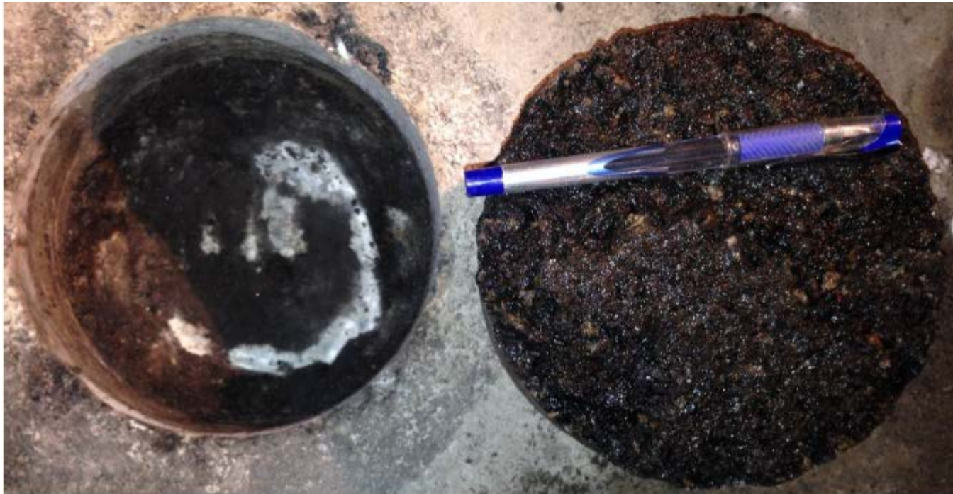
The Bottom of Core 2, Showing Moisture and Stripped Aggregate
