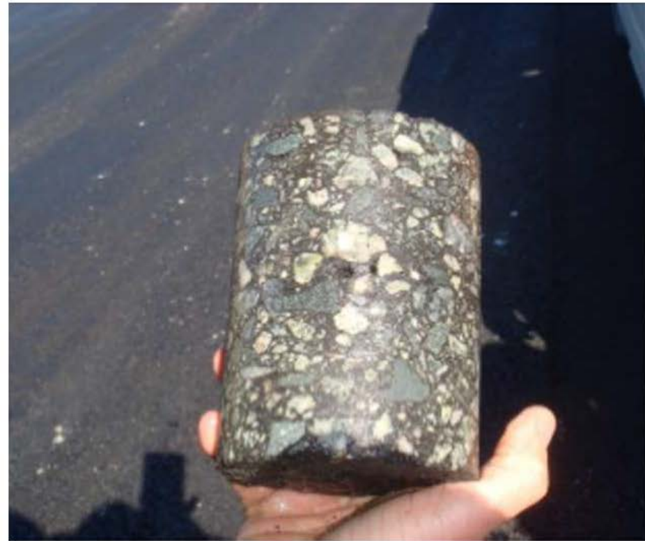
Photo 2: View of the wet core showing some of the voids at the interface.
