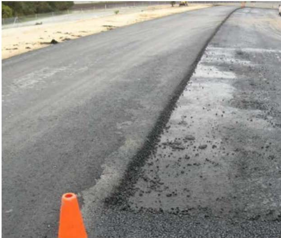
Photo 1: Water seepage from underneath 20mm intermediate mix after rain shower.
