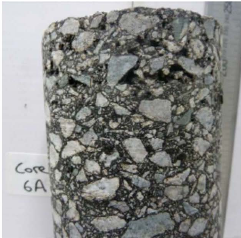
Photo 1: Stripping leading to voided section in core
